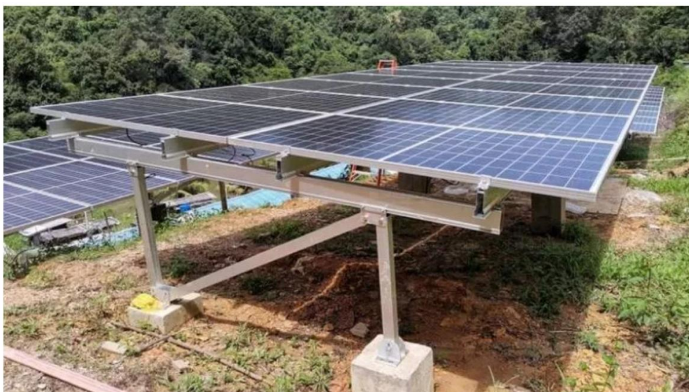
Figure 7: A mounted solar array. The aluminum grid and bars that secure the PV module are prominent [14].
